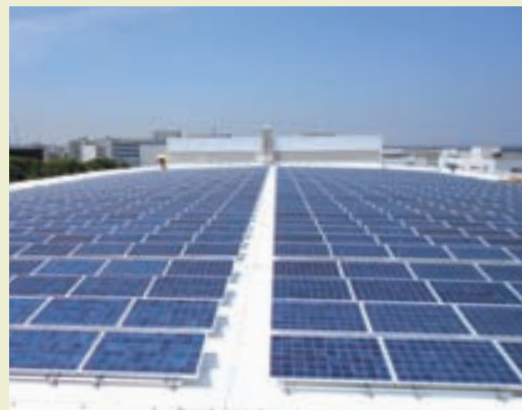
Rooftop solar panels on building at Yokohama Plant
