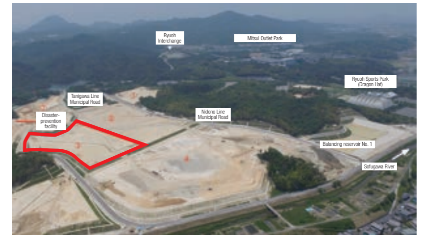
Photo: Area around Shiga Ryuoh Industrial Facility. Planned location of construction of our new factory is indicated with the red line.
