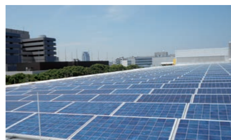
Solar power system at Yokohama Plant
