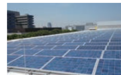
Solar power generation system at the Yokohama Plant
