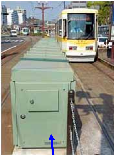
Trolley Voltage Compensation System equipment
