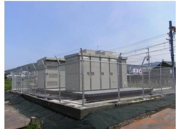
E 3 Solution power storing system
